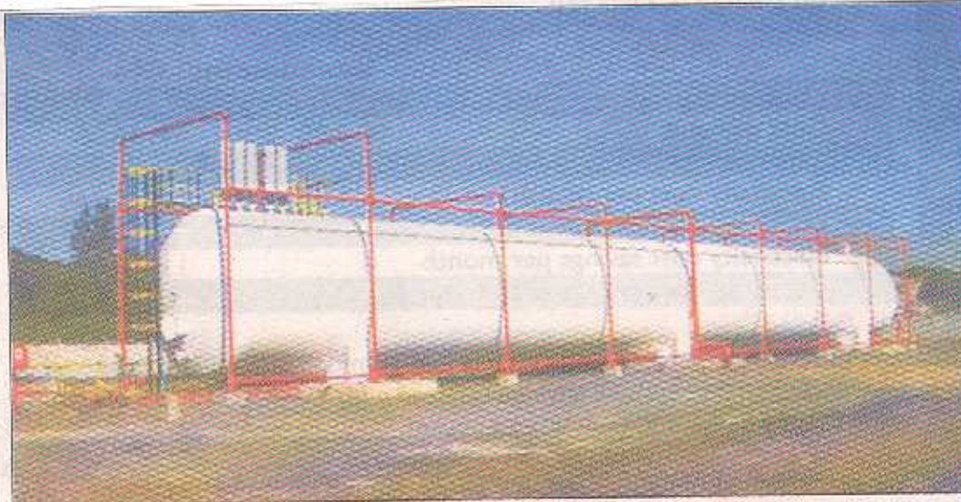
Isegen's giant butane storage tank at Isipingo, Durban recently completed at considerable cost. Butane is pumped from the adjacent Sapref plant and stored partly to offset the annual Sapref's shutdowns.
